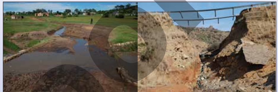
Fig. 3. Road destruction in Botha-Bothe (right) & Quthing during the 2010/2011 floods.
